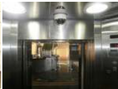
Camera inside the lift
