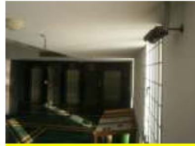
Camera Monitoring all lift entry & exit
