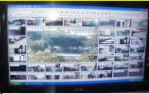
Central Monitoring Station in Computer Facility, JPNATC
