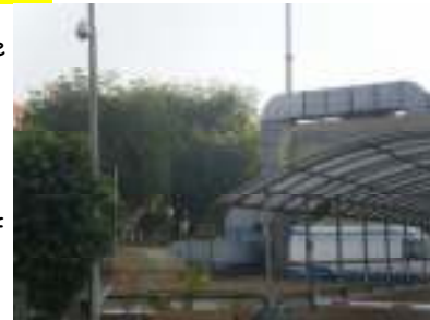
Outdoor Camera for parking area
